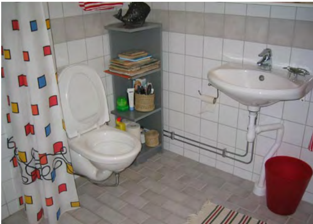
Figure 4.3.4.2 Urine-diverting flush toilet installed in a home in Kullön, Sweden.
