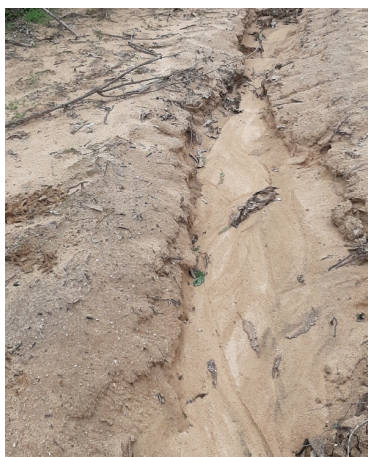
Figure 3.4.4.2 Soil erosion, with loss of topsoil, caused by road construction.
